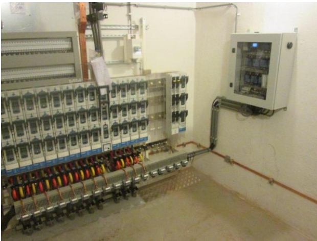
Fig 6 : Low voltage switchgear and measurement cabinet
