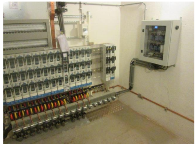
Figure 4 : Low voltage switchgear and measurement cabinet
